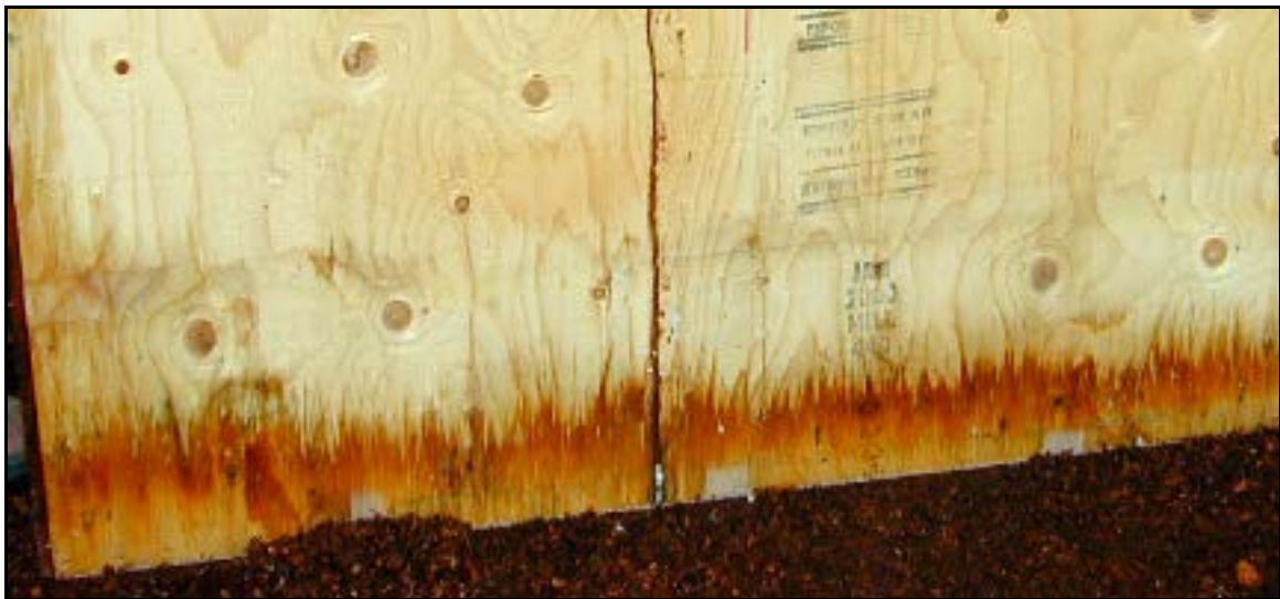
Photo 1 – Backside of Removed Panel Siding Reveals the ‘Wicking’ that Can Occur When a Porous Material Is Installed Tight (No ‘Capillary Break’) to a Horizontal Base Flashing
