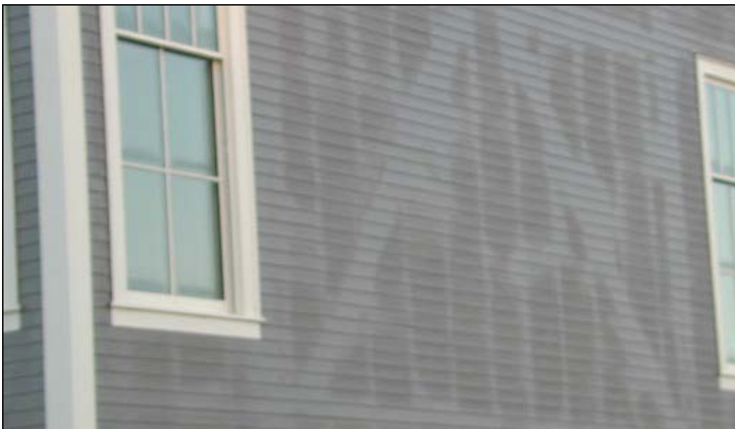
Photo 2 – Morning Dew Forms Only at Fiber-Cement Siding Areas Not Warmed by the Underlying Steel Framing (Coe Elementary School, Seattle)
