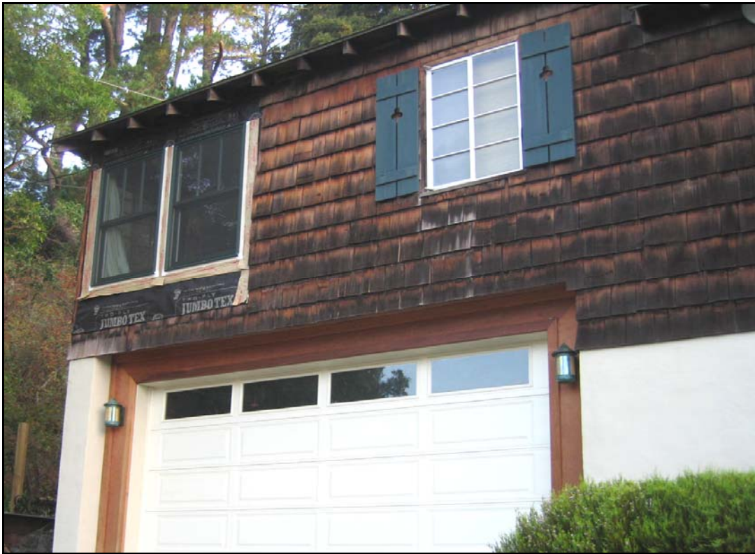
Photo 1 – Owner Is Replacing the Original Aluminum Windows (at Right) with New Metal-Clad Wood Windows (at Left). Note the Severely Deteriorated Redwood Shakes
