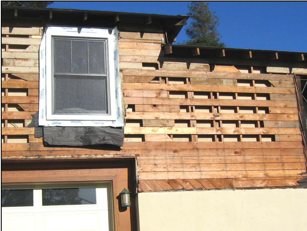
Photo 2 – However, Removal of the Deteriorated Redwood Shakes Reveals No Water Damage at the Wood Board Sheathing or Stud Framing
