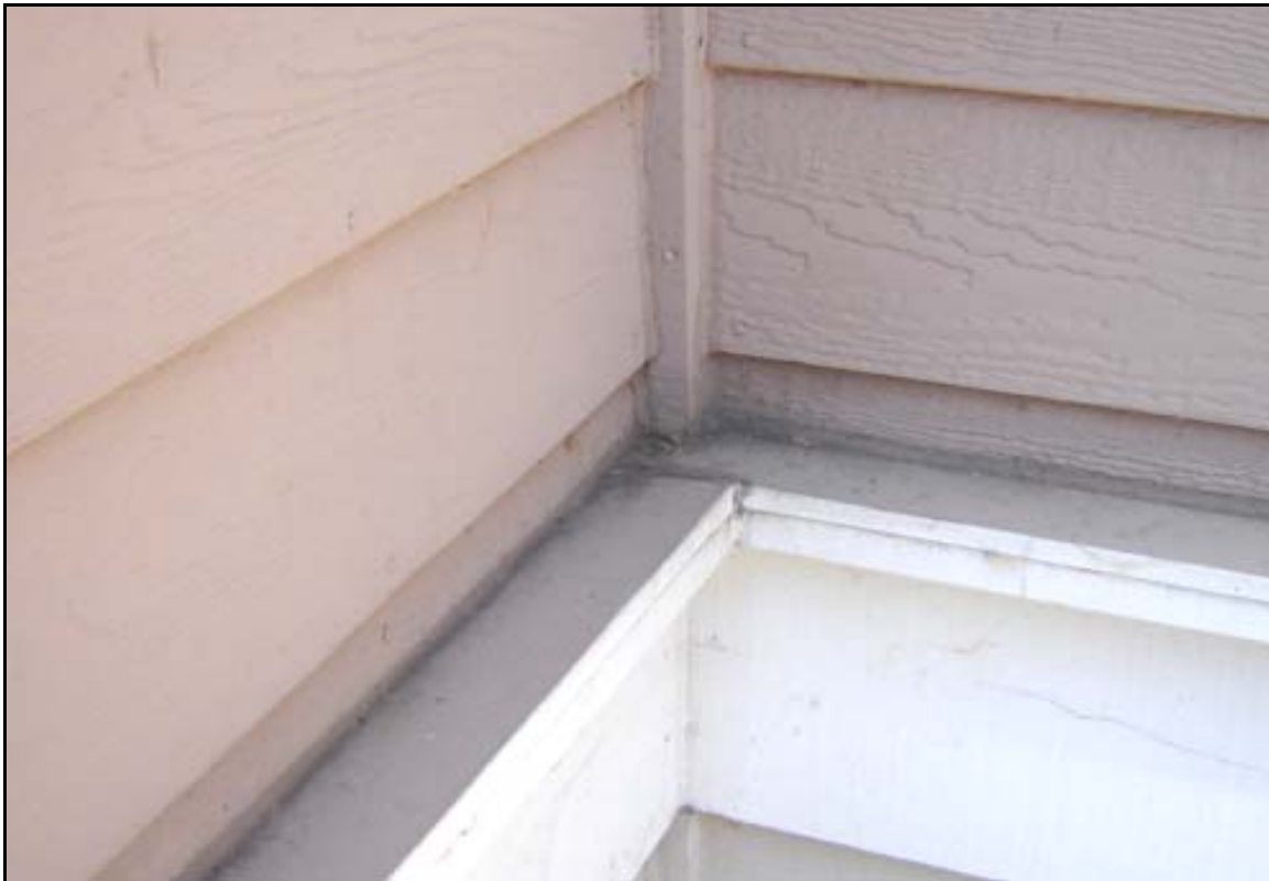
Photo 1 – Is this metal flashing installed in such a manner so as to prevent moisture from entering the wall or to redirect it to the exterior?
