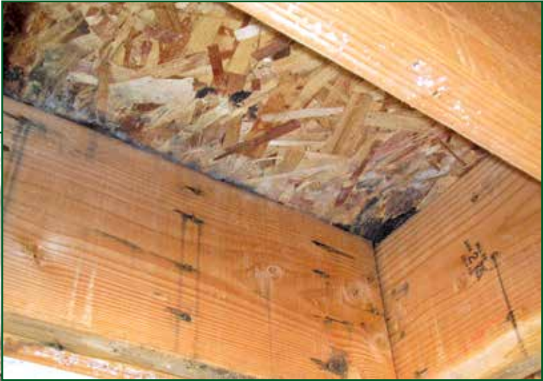
Photo 9 – Soffit removal below another deck reveals evidence of water seepage from above.
