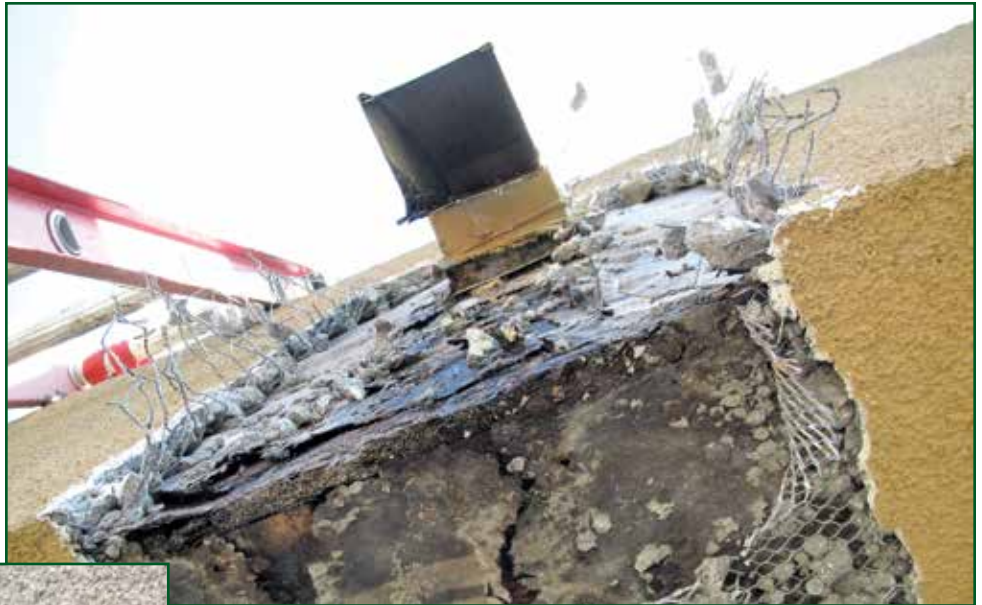
Photo 3 – Seepage from under the scupper box, likely from a hidden pool of trapped water.
