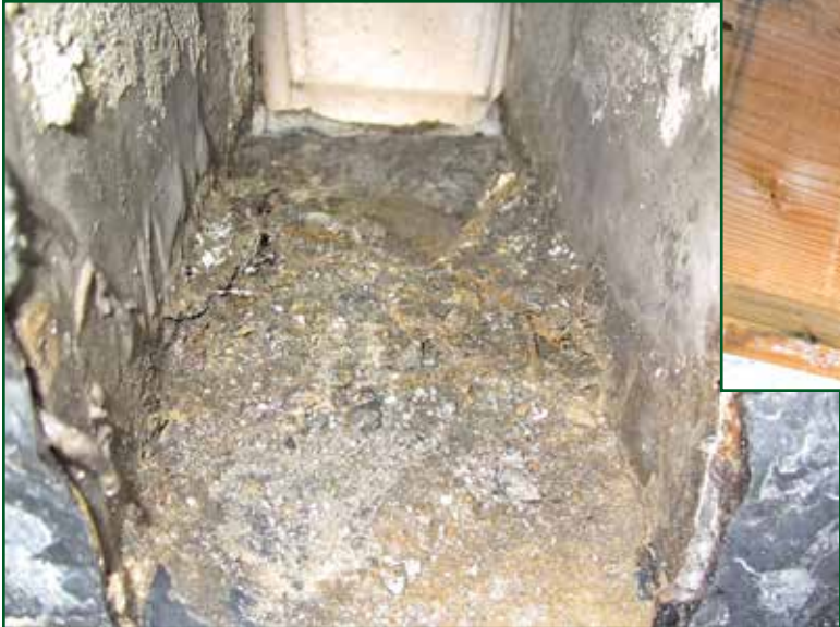
Photo 8 – Concrete debris within the scupper’s throat impedes positive drainage.
