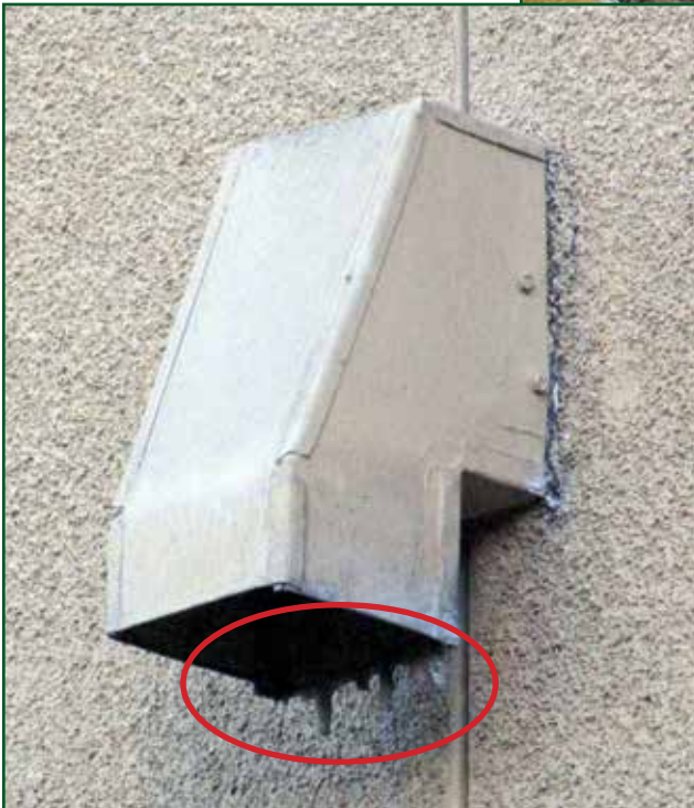
Photo 2 – “Concrete stalactites” are evidence of slow seepage of ponded water.
