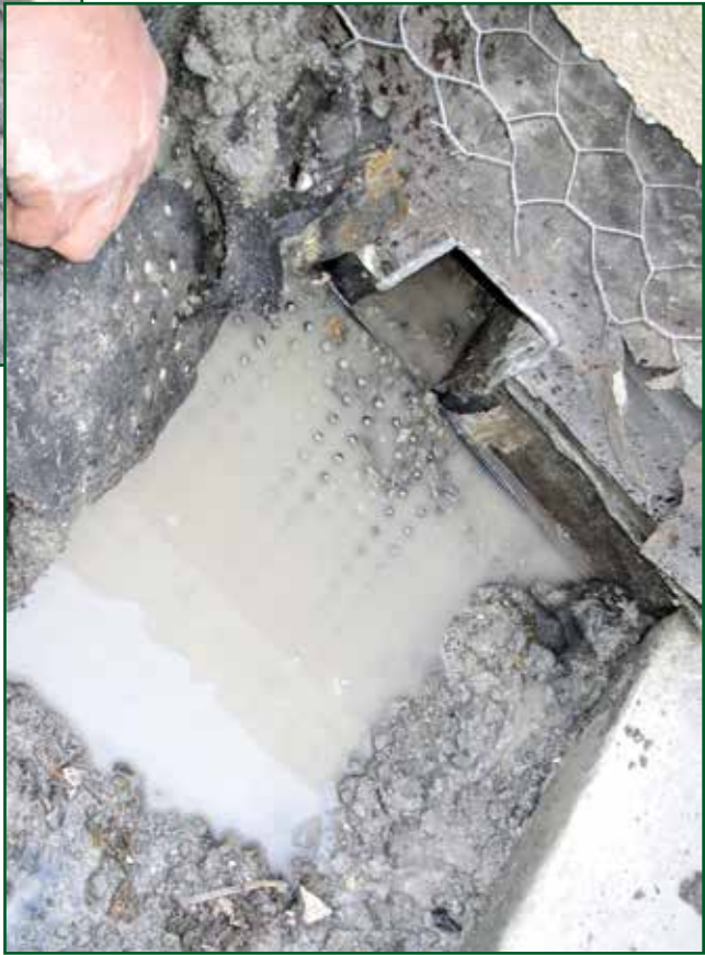
Photo 7 – Water ponds due to negative slope and other construction deficiencies.
