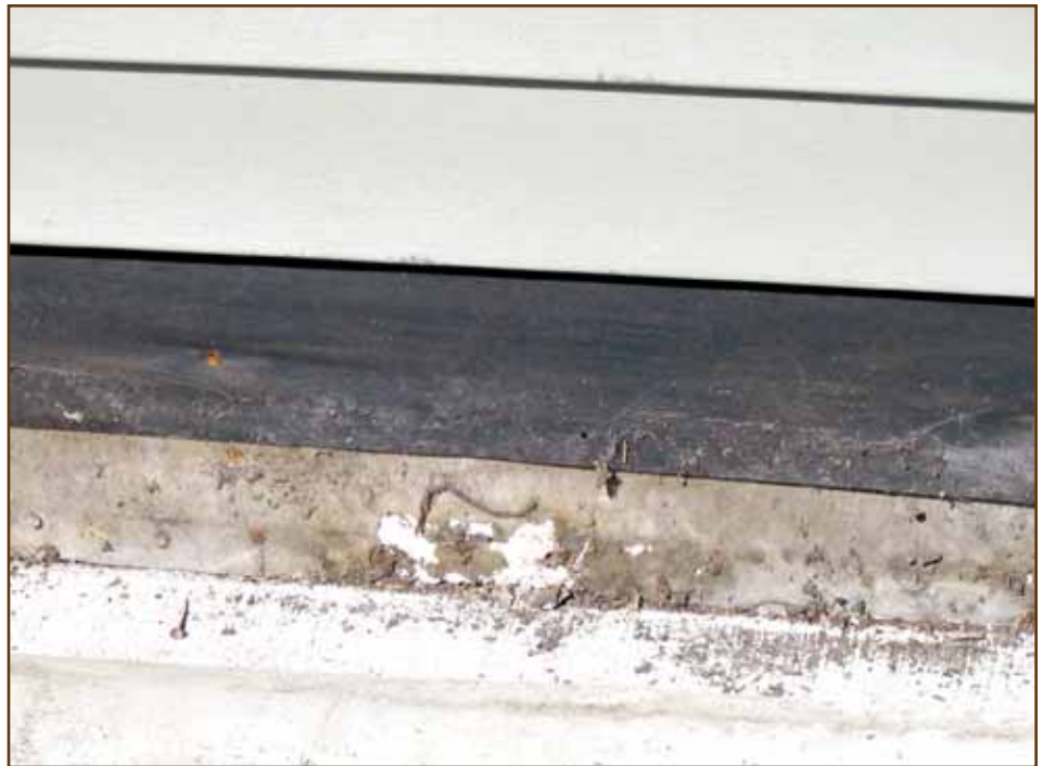
Photo 4 - Water and mold damage to gypsum sheathing terminating at hardscape
