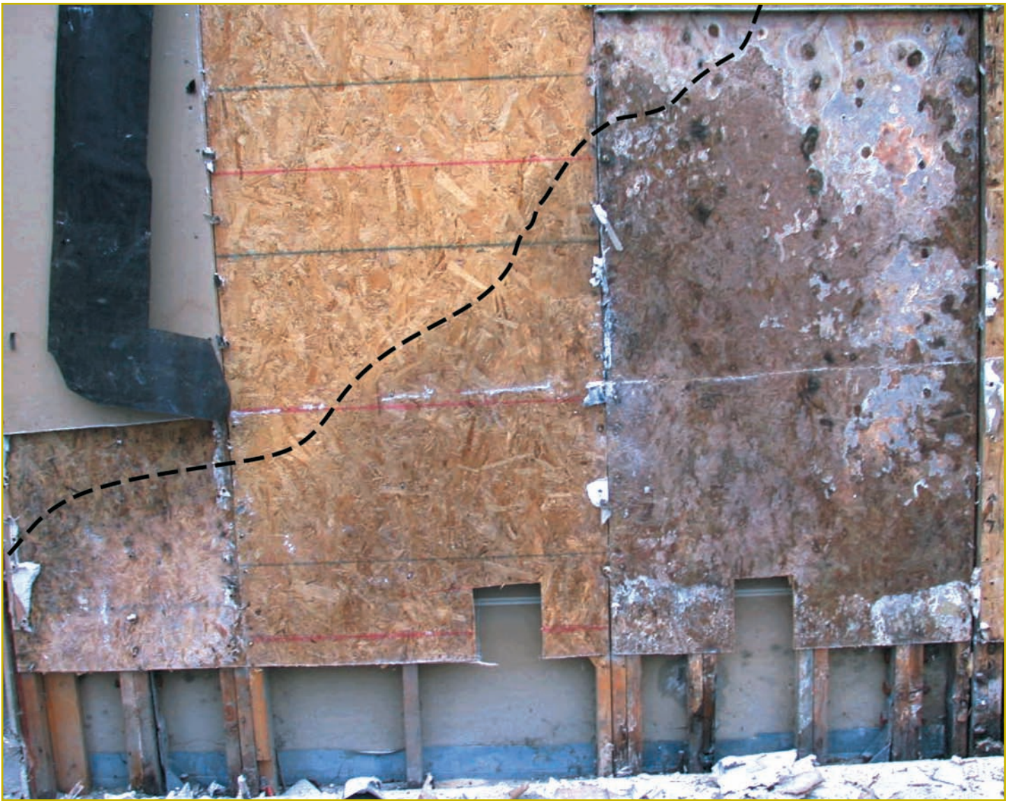
Photo 3 - Undamaged center panel is sandwiched by two white-rotted panels. (The dashed line traces the upper limit of the migrating water.)
